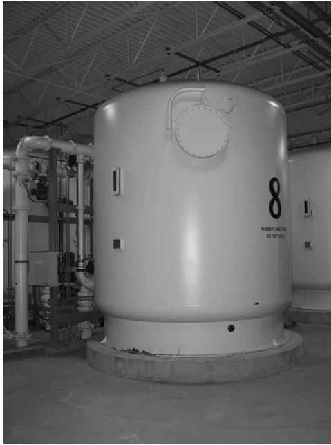
Figure 3. Ion exchange vessel and connecting piping header.
