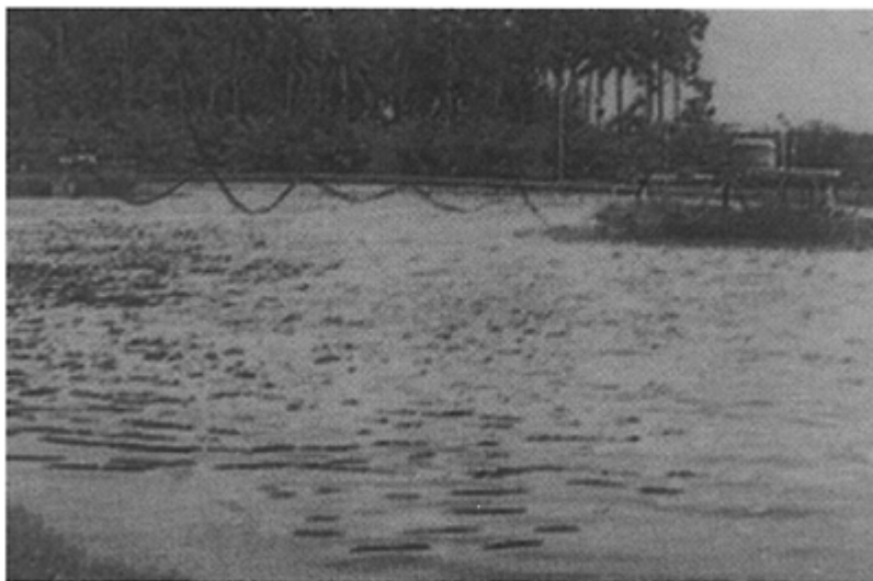
Figure 8 An aerator system installed to accelerate BOD reduction at the aerobic pond. (Courtesy of Malaysian Palm Oil Board.)
